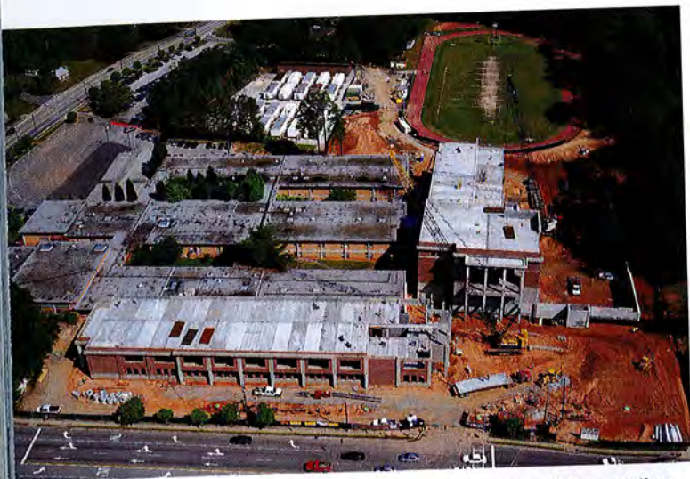
During construction of the new Tucker High School, the existing school remained in service, leaving minimal staging area and requiring just-in-time delivery and erection of precast components
